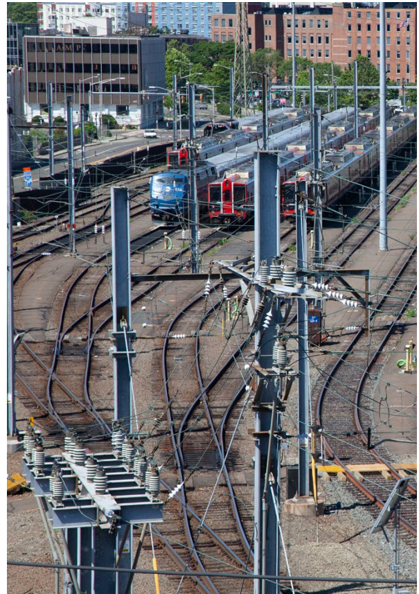
Electric Infrastructure in Stamford, CT
