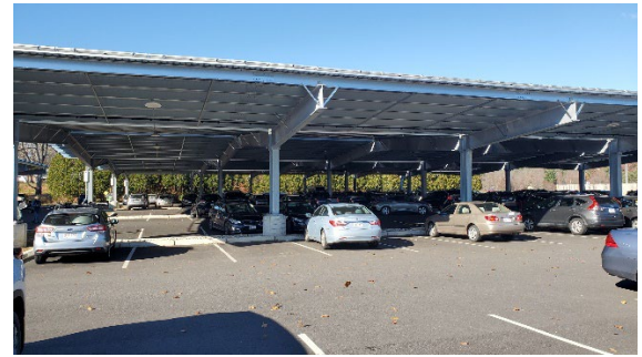
Ground-Level Solar Canopy at UMass Amherst
