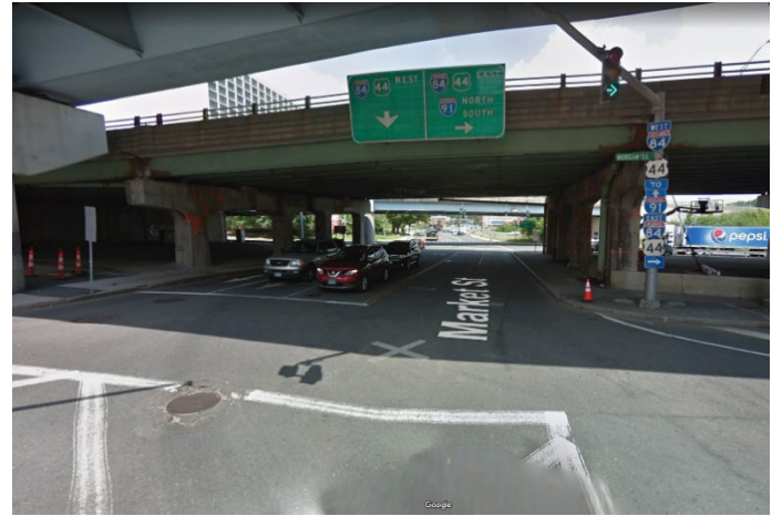
Sample Facilities in the Vicinity of I-84 in downtown Hartford (Source: Google StreetView)
